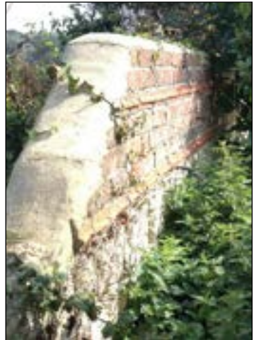
St Helen's House: part of the north wall
